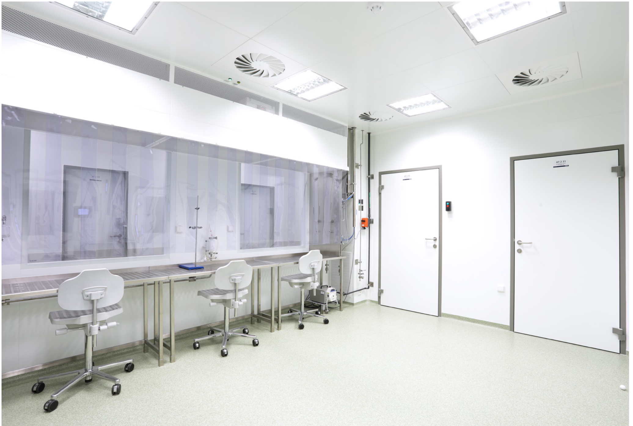
Virology Department on the 2nd Storey Above Ground of The Bioveta Novelty Hall (BNH) | Bioveta a.s, Ivanovice na Hané | Czech Republic | 2018
