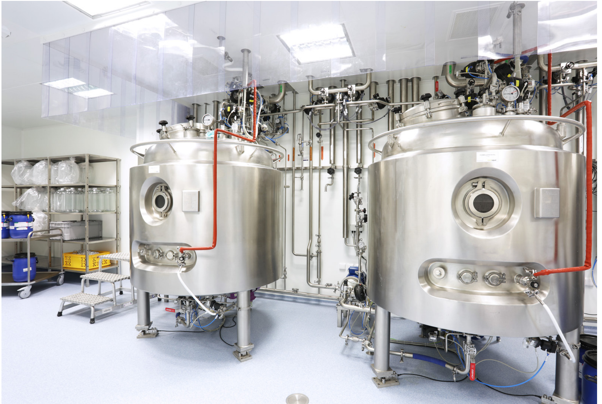
Virology Department on the 2nd Storey Above Ground of The Bioveta Novelty Hall (BNH) | Bioveta a.s, Ivanovice na Hané | Czech Republic | 2018
